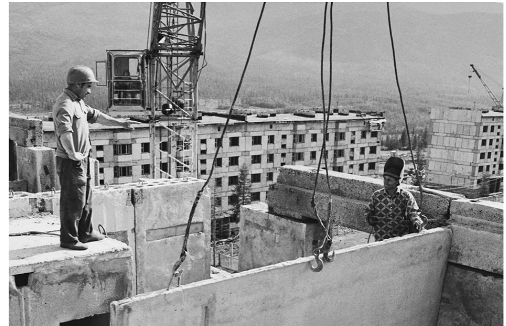
23. Construction of the settlement of hydro-builders of the Kolymsky HPP Sinegorye. Nikolai Tishukov (left) and Viktor Balkhanovsky at the assembly of a residential building. 1978
